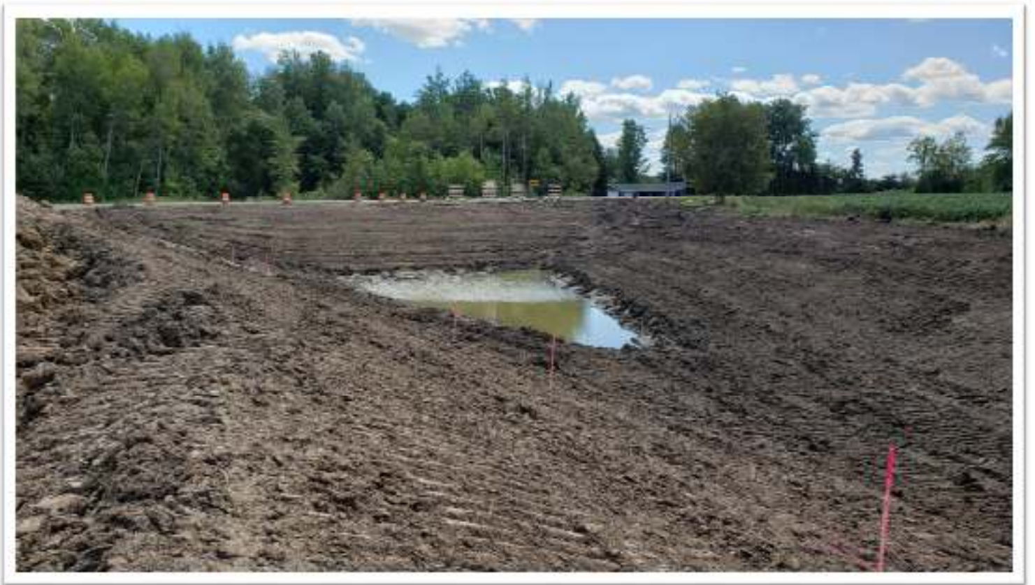
Storm water retention pond
