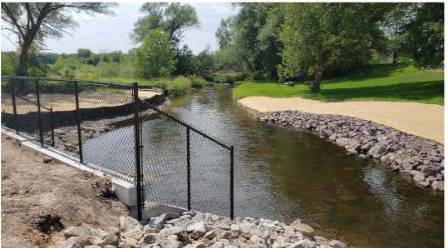
West bank safety fencing
